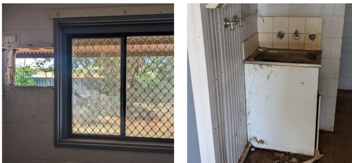
Figure 13. Hole in wall and broken laundry sink. Images. Liam Grealy
