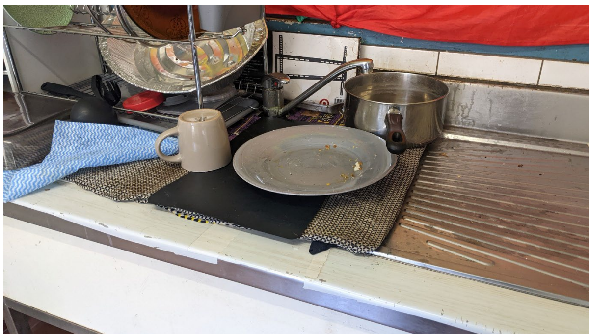
Figure 15. Broken sink and householder work-around. Image. Liam Grealy
